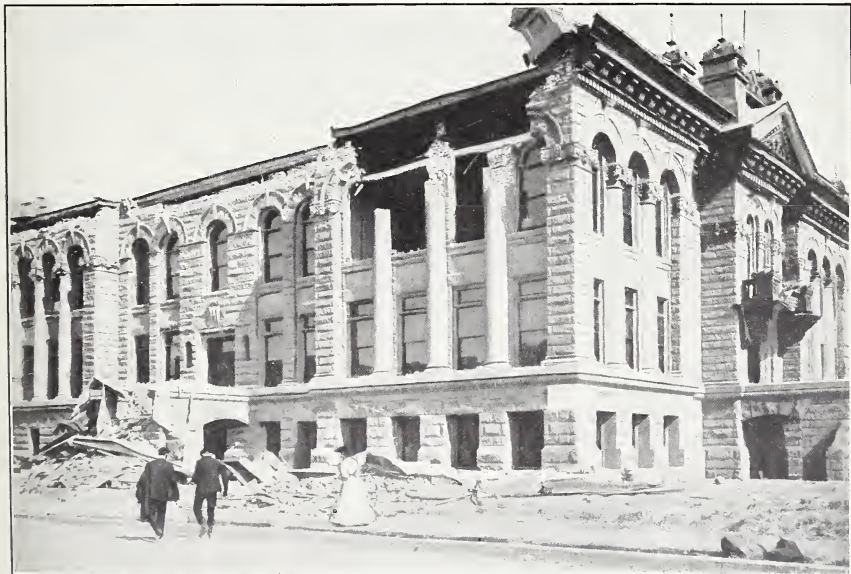
B. EARTHQUAKE WRECK OF NEW HALL OF JUSTICE, SAN JOSE, BUILT ON ALLUVIAL SOIL.
